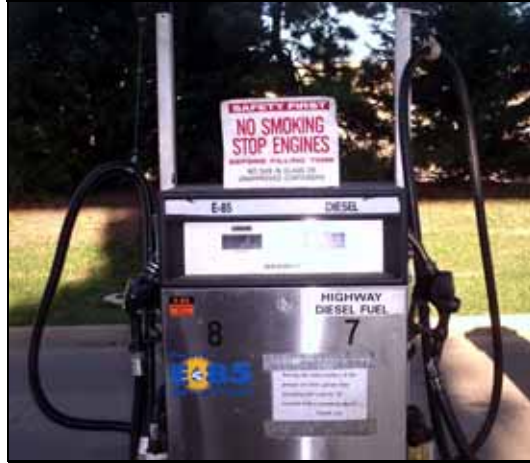
B20 Dispenser – Arlington pumps B20 and E85 from this dispenser at its Shirlington facility.
